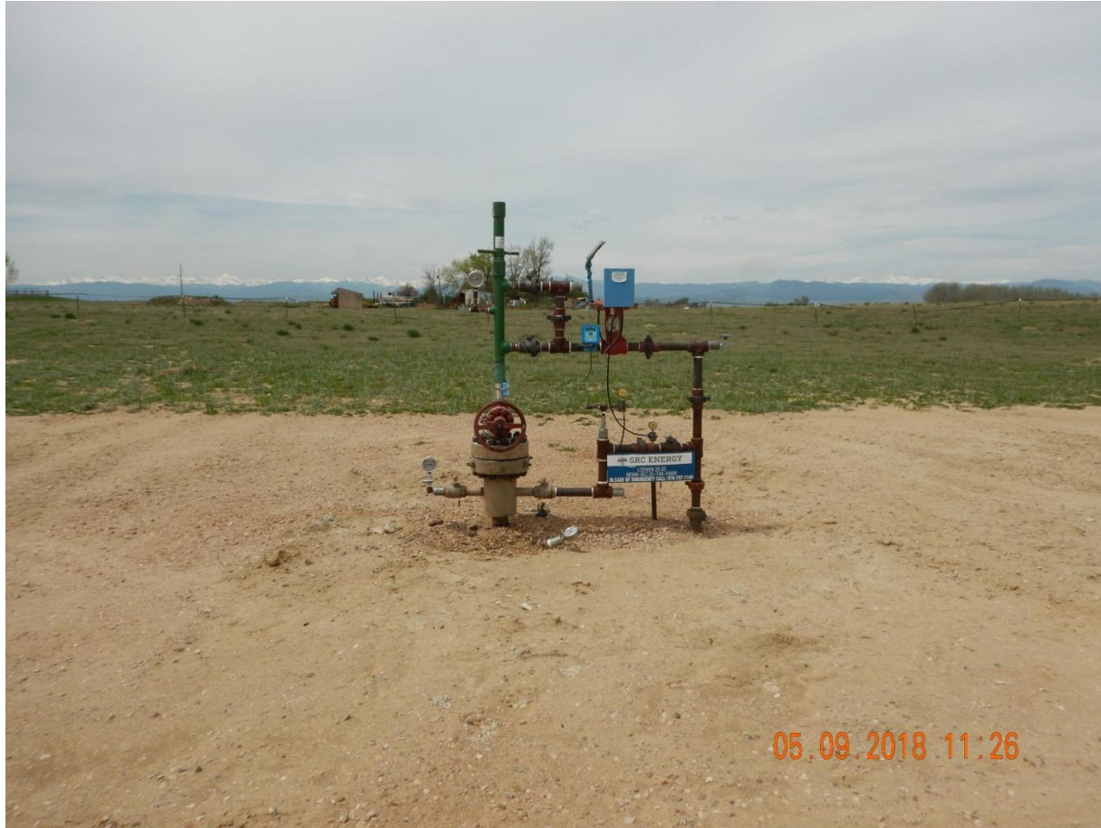
Photo 1. Photo taken from the central location, facing West. Operator plugged 4 of 5 wells on location. Location appears to be in overall good condition regarding 1000 Series rules and regulations.
