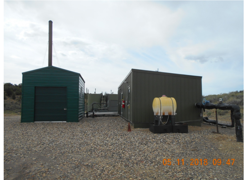
Pump housing and Generator housing
