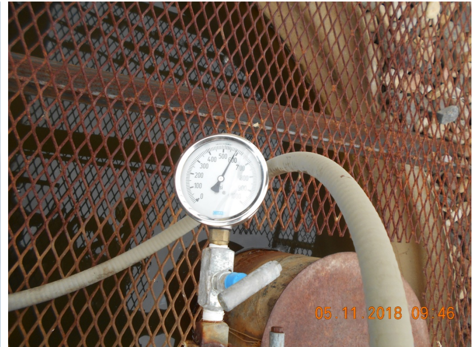
Casing gauge on wellhead
