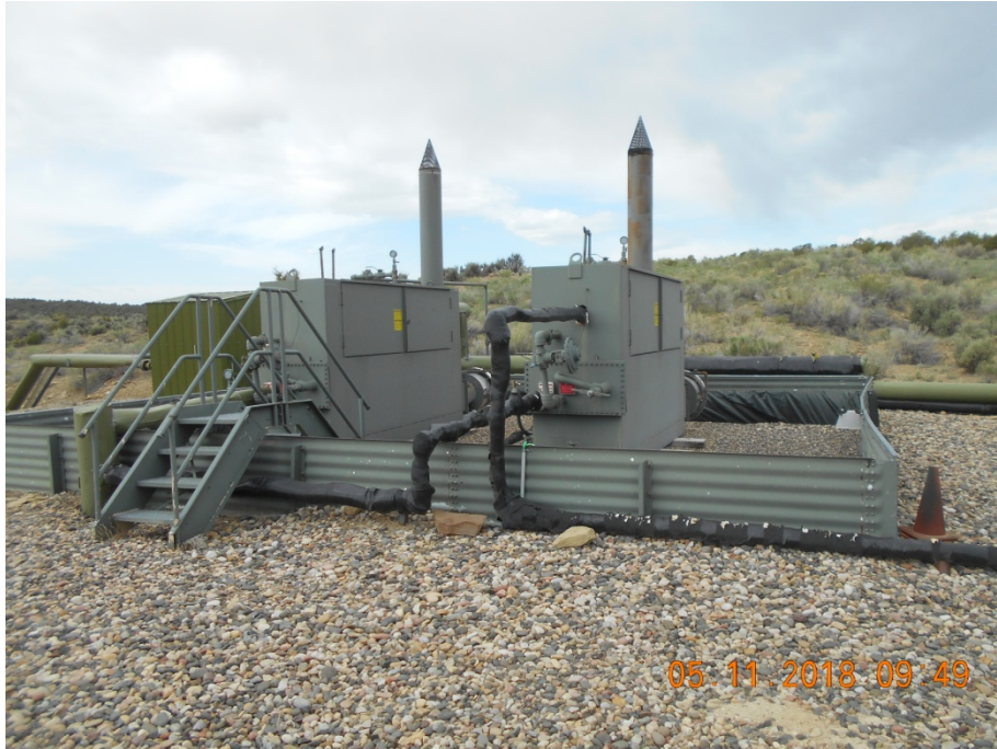
Separators and meter housing
