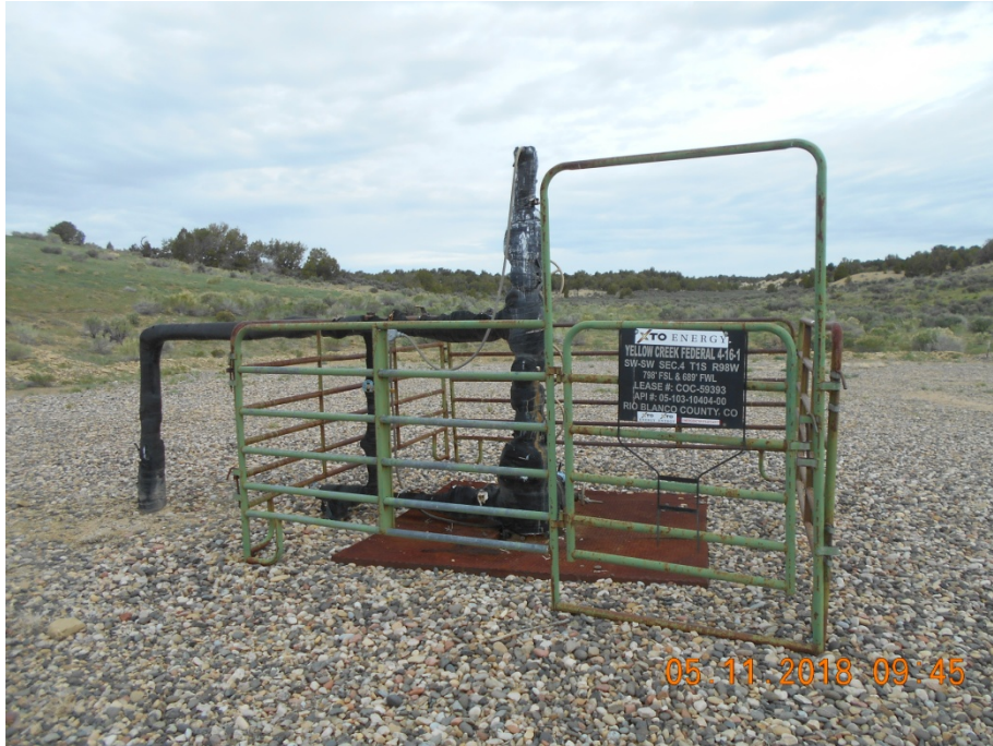
Injection wellhead with fencing and sign
