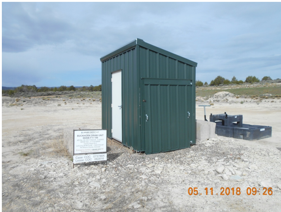
Injection wellhead housing with sign
