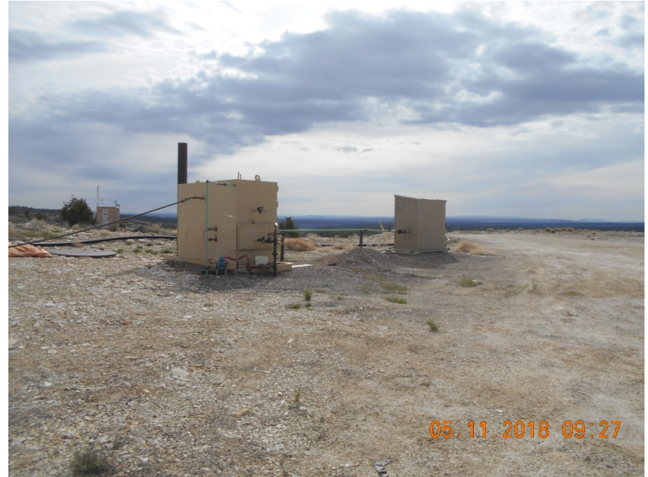
Separator and Meter Housing
