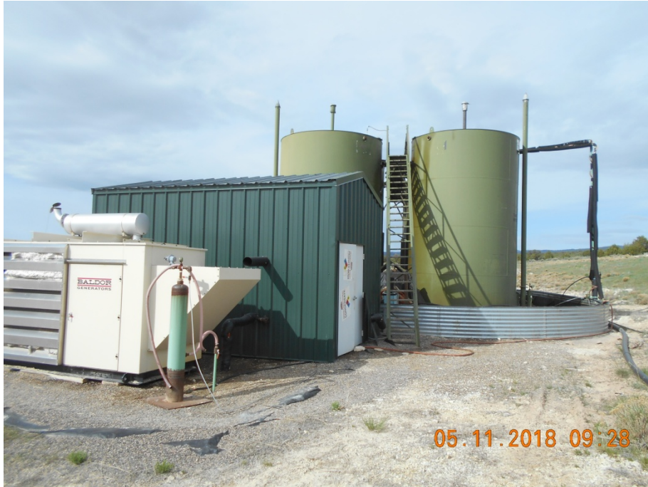
Tank Battery , Pump housing and Generator
