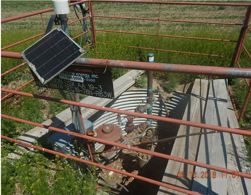
Photo 1: Wellhead, looking N
