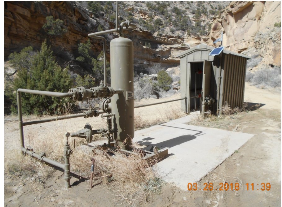
Scrubber and Meter housing
