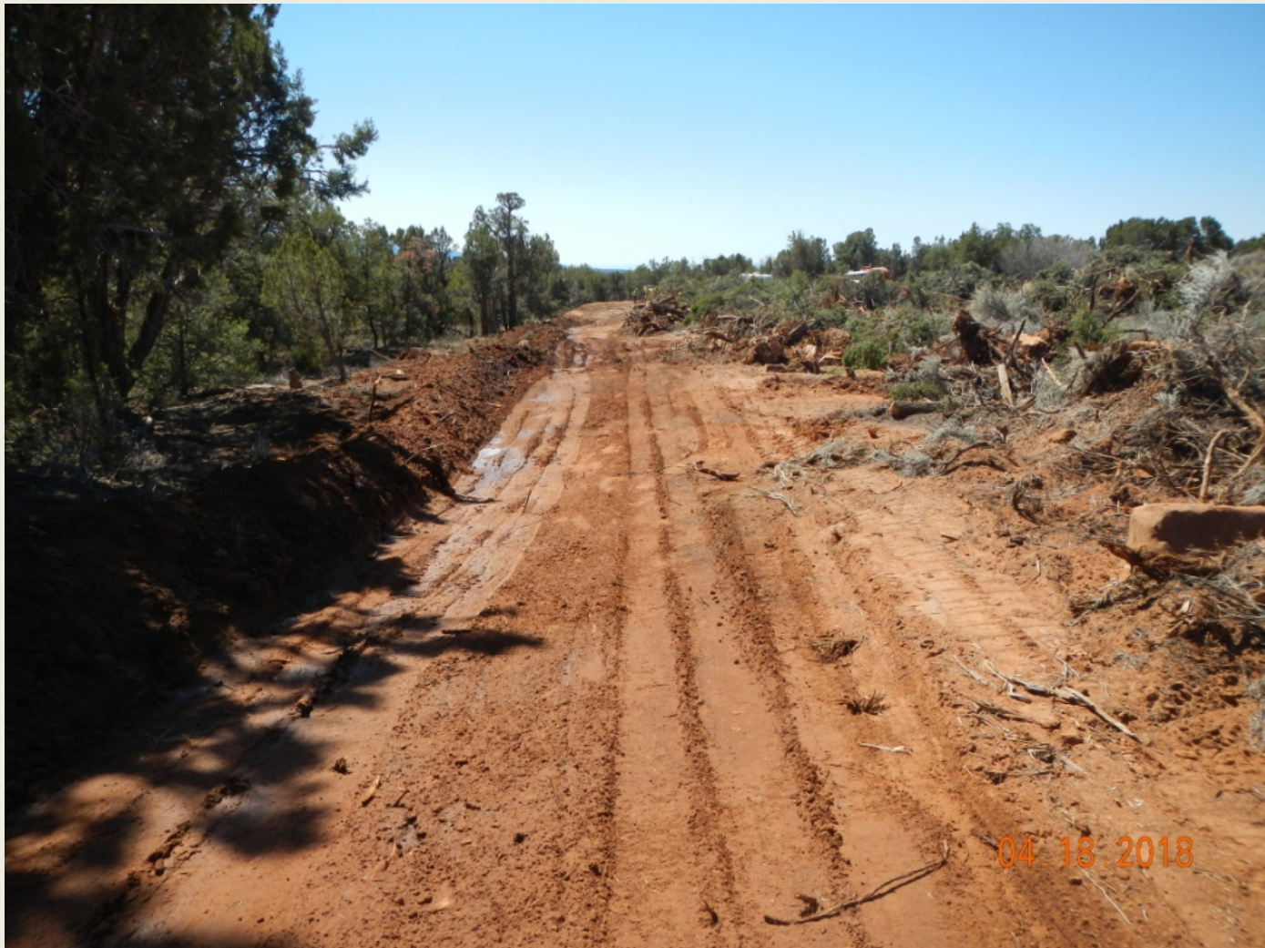
Photo 2. View of the edge of the project area from the northeastern corner facing southward. Vegetation removal is occurring and berms are being constructed. Per communication with onsite management, berm compaction will be completed this day.
