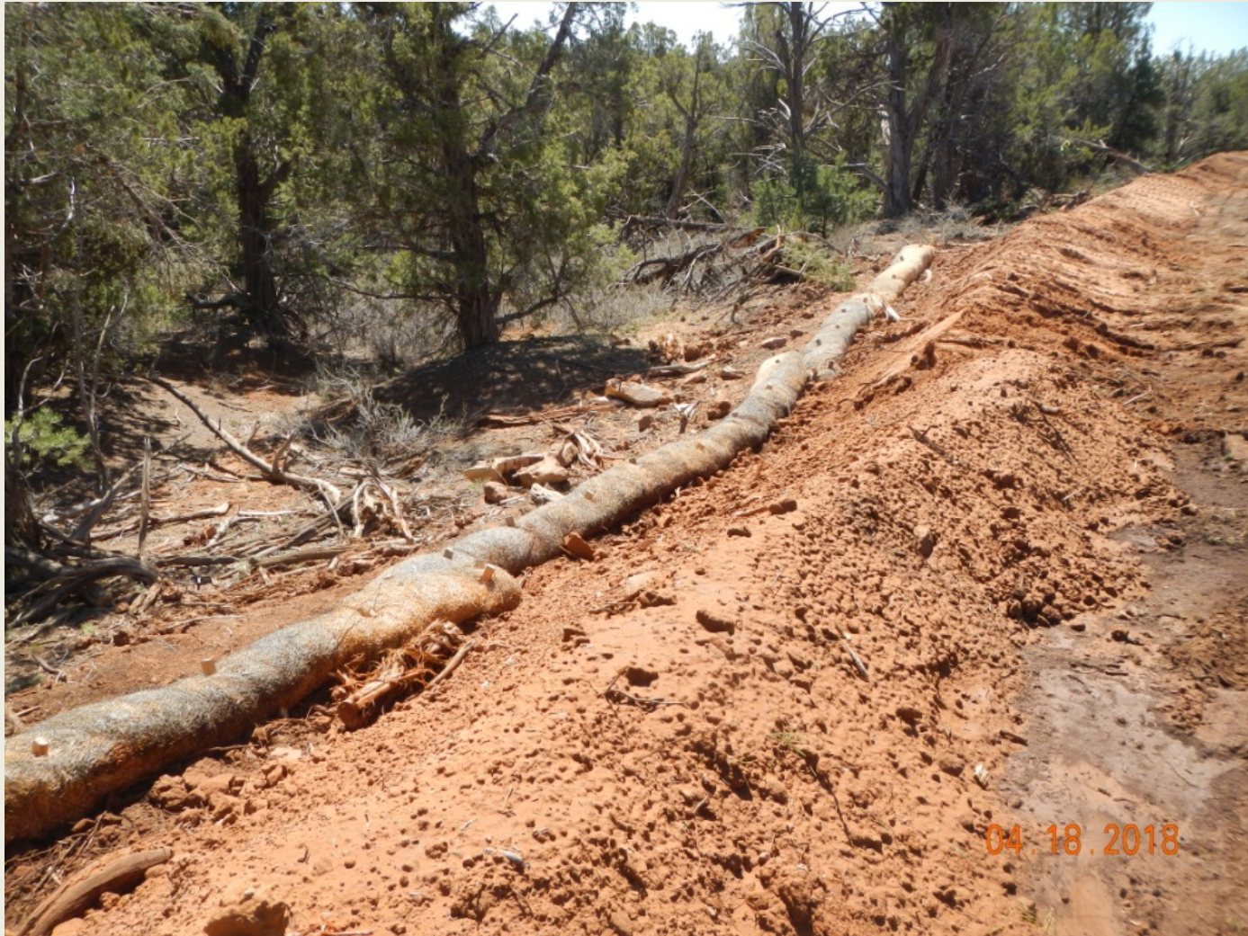
Photo 4. View of wattles in the eastern project area. Wattles should be placed outside of disturbed soils to prevent runoff.
