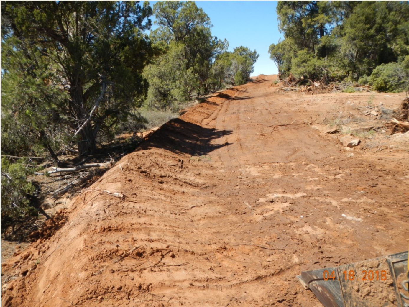
Photo 5. View of the southeastern edge of the project area. Berms are properly compacted here. Vegetation on the well pad is in process of removal.
