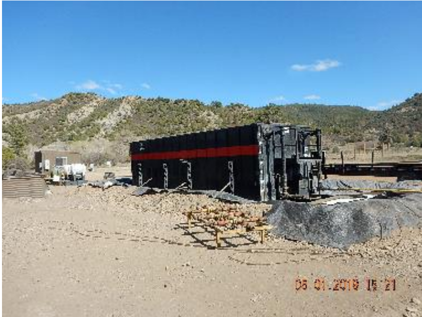
Photo 3: Flow back tank in lined and bermed containment.
