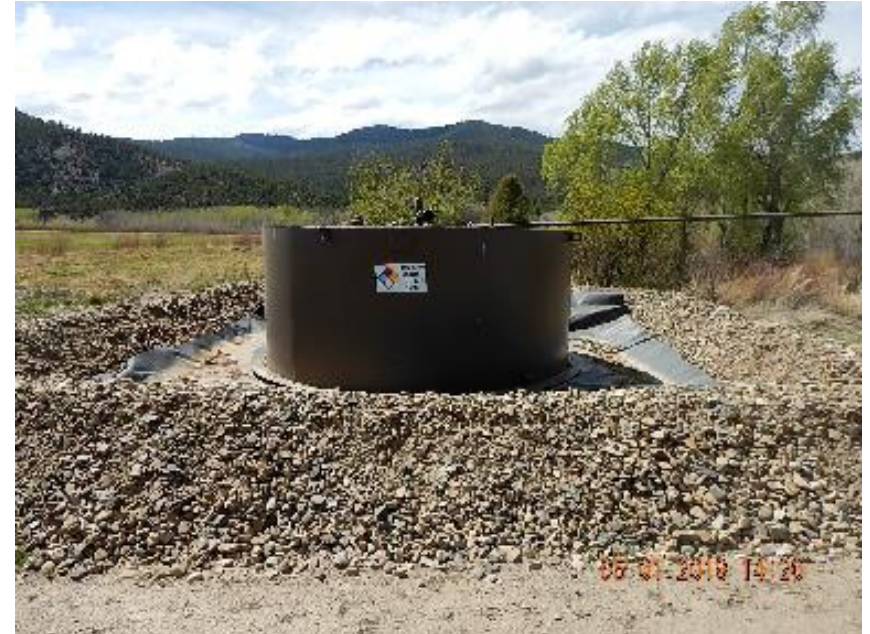
Photo 6: Open top with labels installed.
