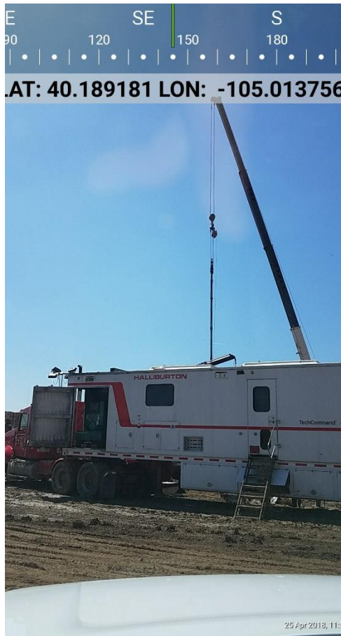
Photo 1 Lubricator and Data Shack
