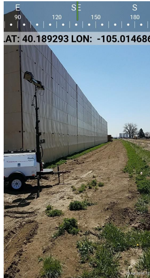
Photo 5 Location Sound Wall and Ditch on West Side
