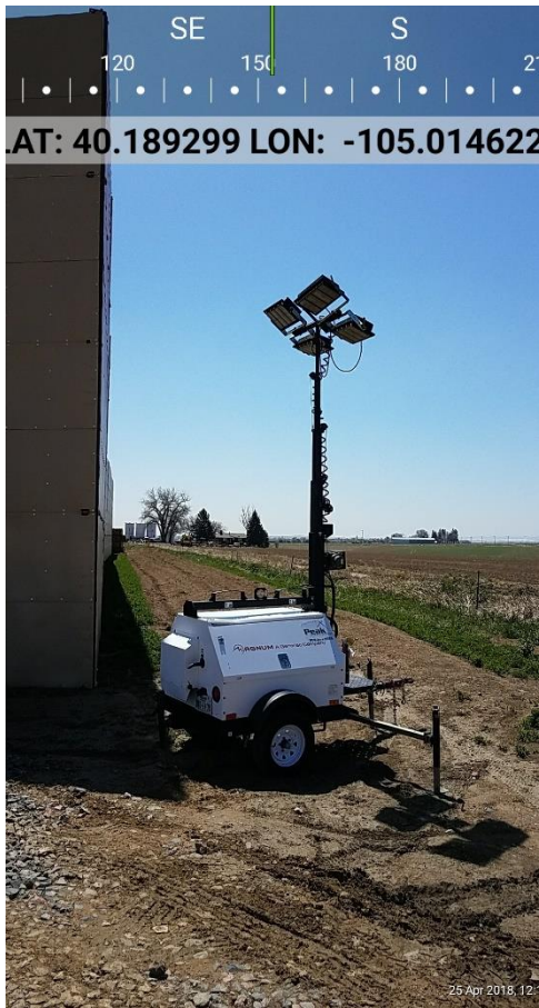
Photo 4 LED Light Tower
