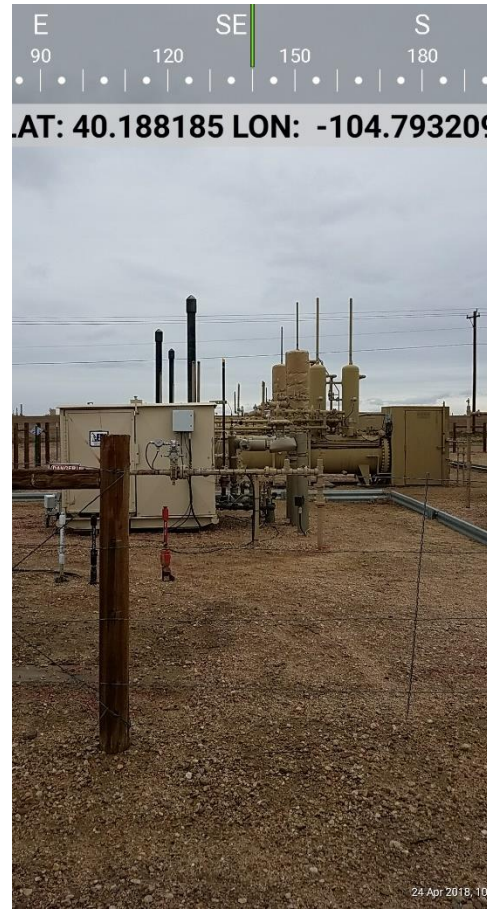
Photo 8 Gas Meter Runs
