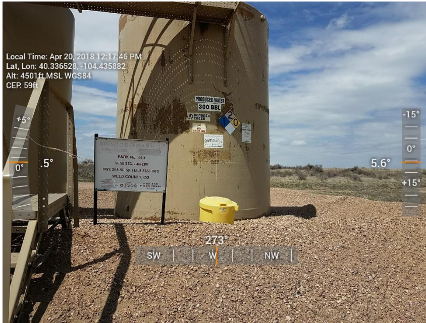
Tank battery signage
