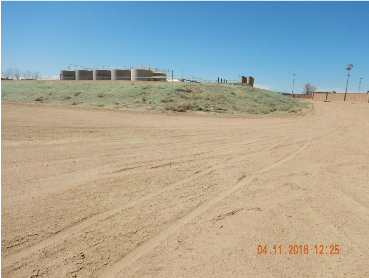
Photo 6. Photo taken east of the location, facing West. The fill north and east fill slopes have not been stabilized. Erosion blanket netting no longer in proper functioning condition.
