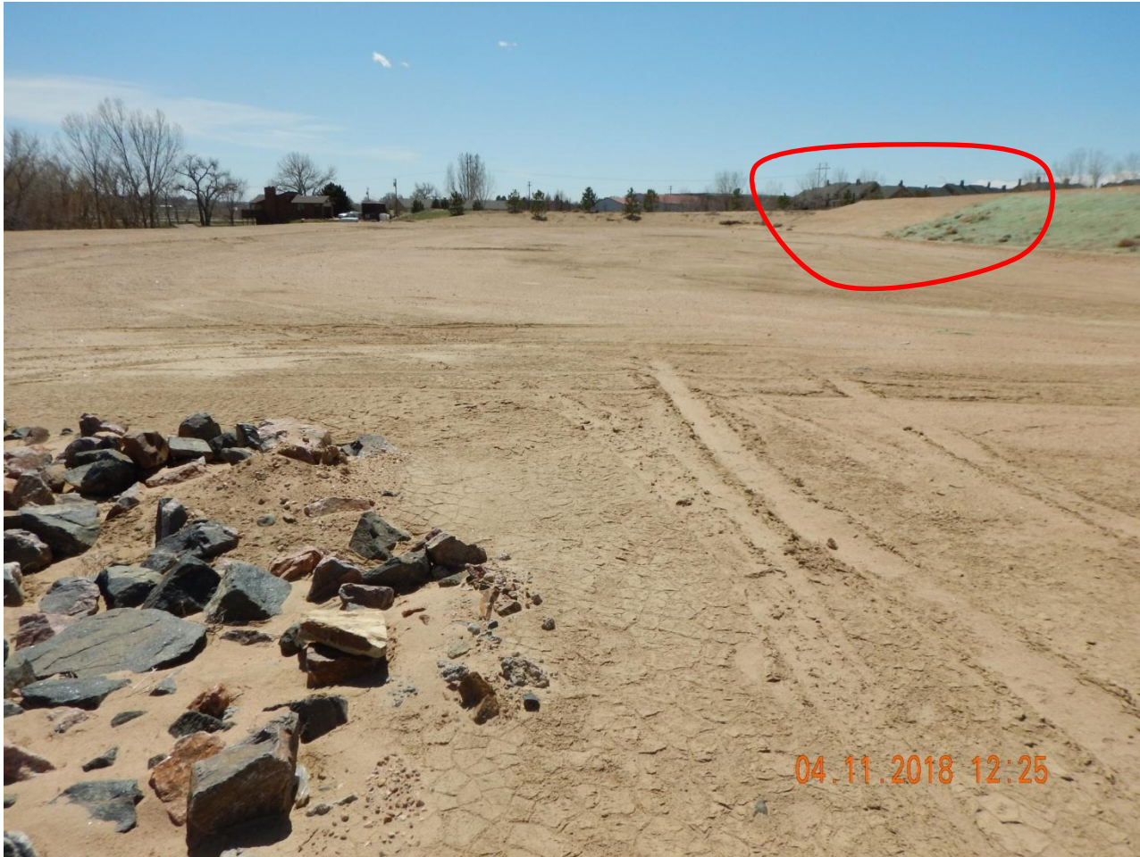
Photo 7. Photo taken east of the location, facing South. Photo illustrates the southeast fill slopes has not been stabilized.
