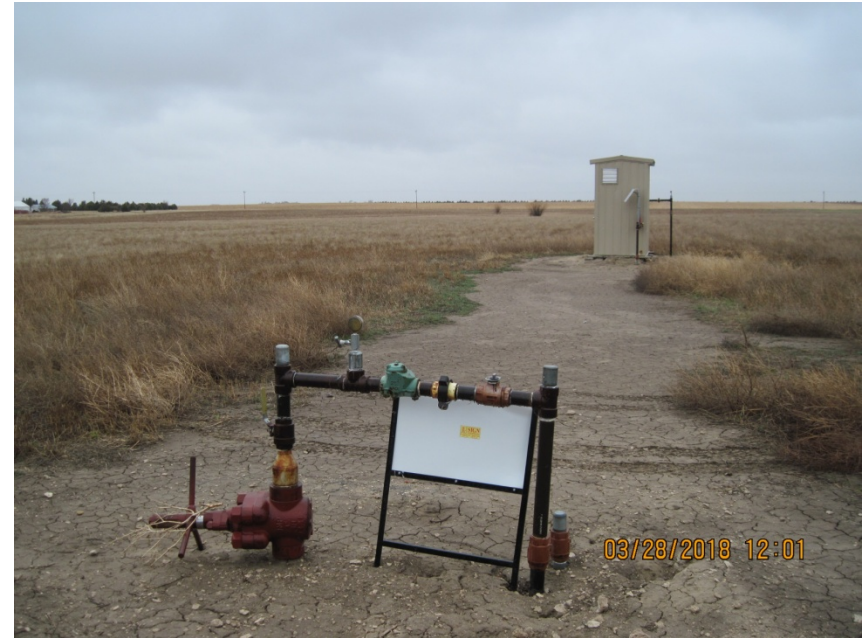
2. Meter shed & wellhead
