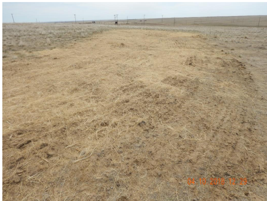
Photo 4: Photo taken from the east end of the location, facing south. Photo shows areas appear to have had additional reclamation activities conducted. Area appears to have been reseeded and stabilized with a mulch.
