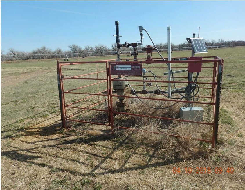
Photo 1: Wellhead, looking E
