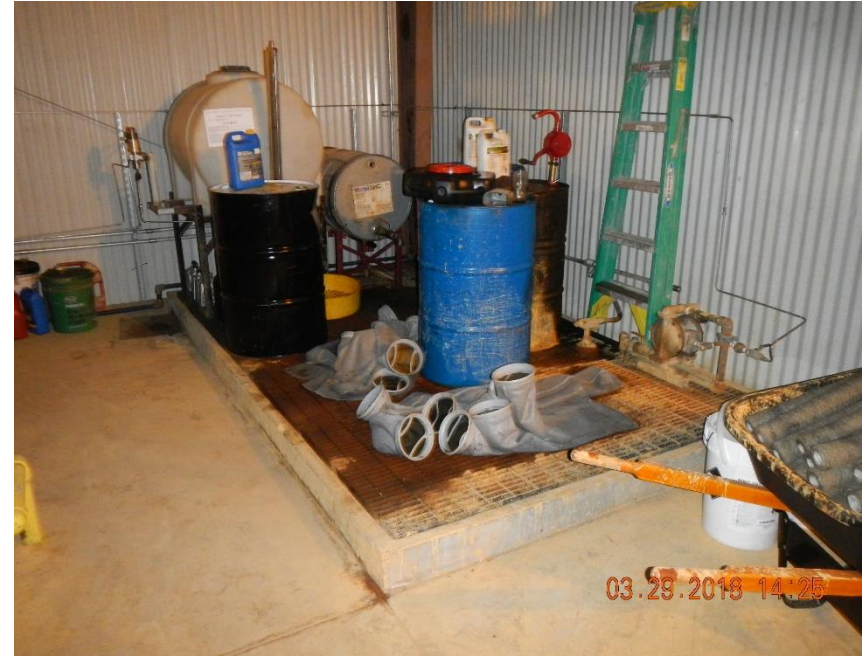
Chemical storage with secondary containment.
