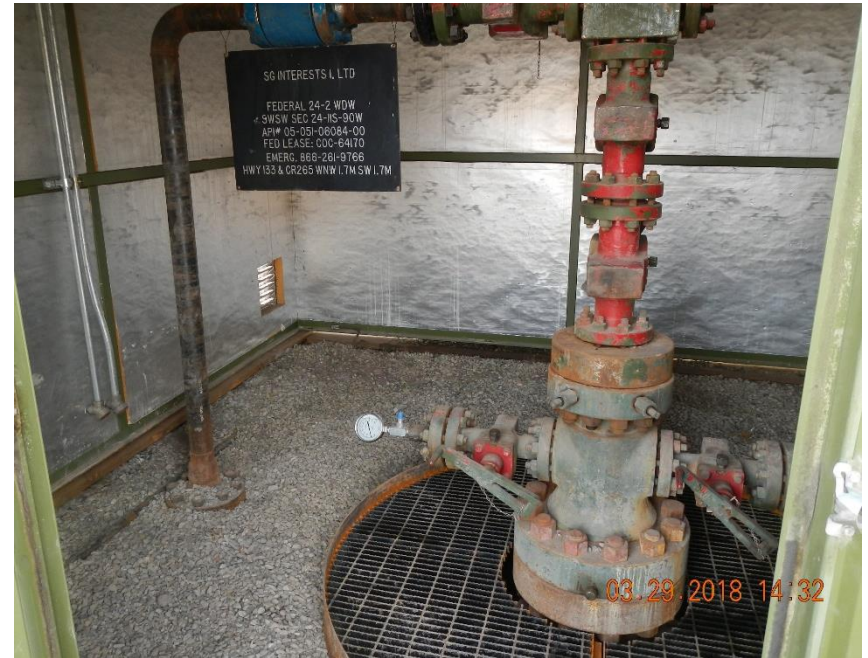
Federal #24-2 WDW well head.
