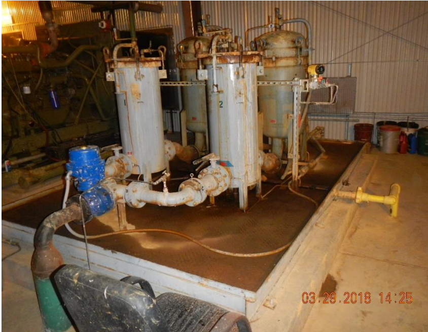
Filter assembly on secondary containment.
