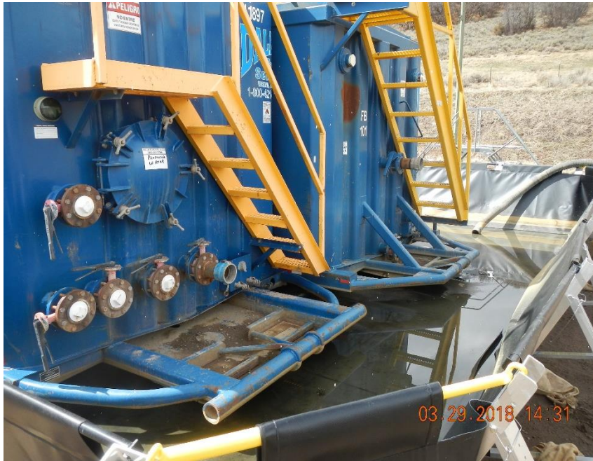
Frac tanks have labels and placards.
