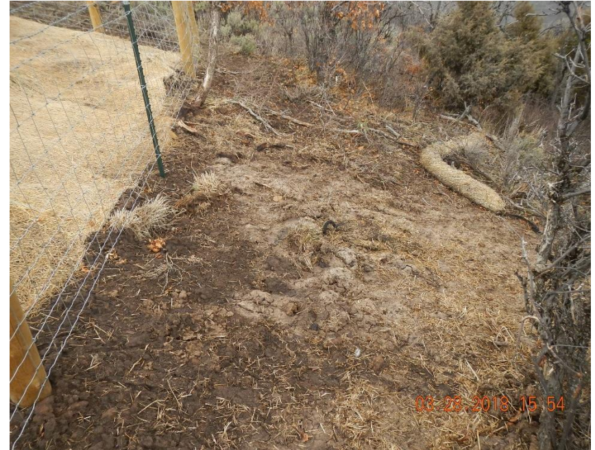
Wattles on downhill side of project area have been destroyed/require attention.
