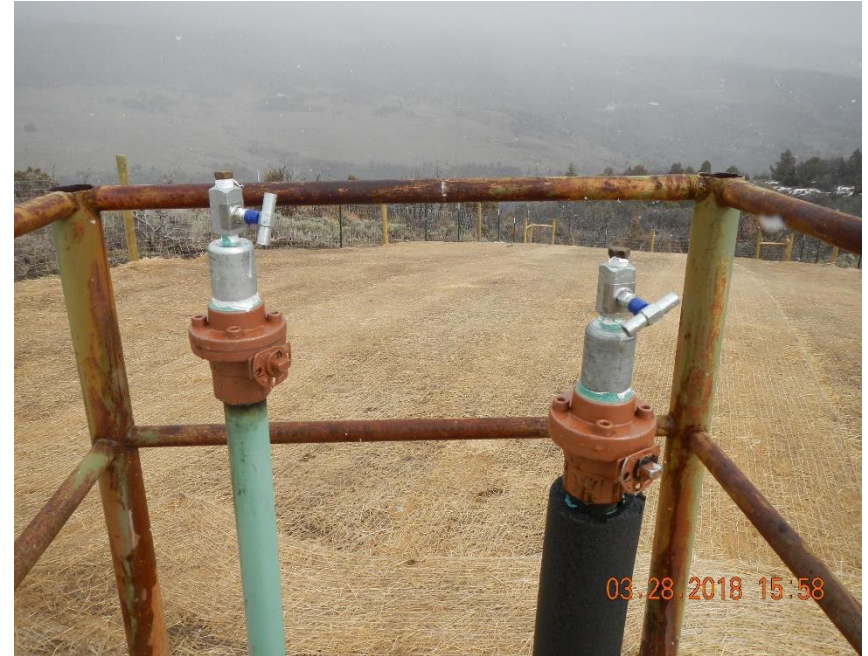
Water and gas risers.
