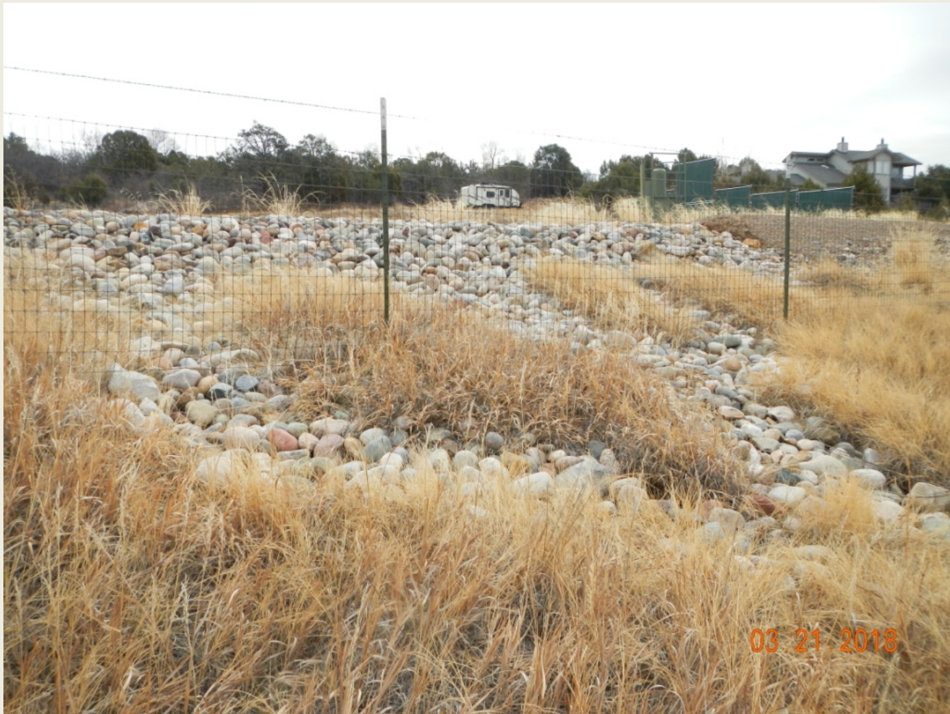
Photo 6. View of erosion controls in the western project area, appear to be functioning at this time.
