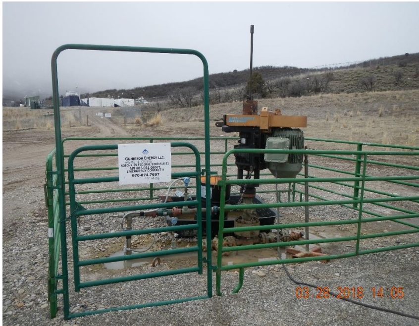
Hotchkiss Federal 1289 #18-31 well head and pump.
