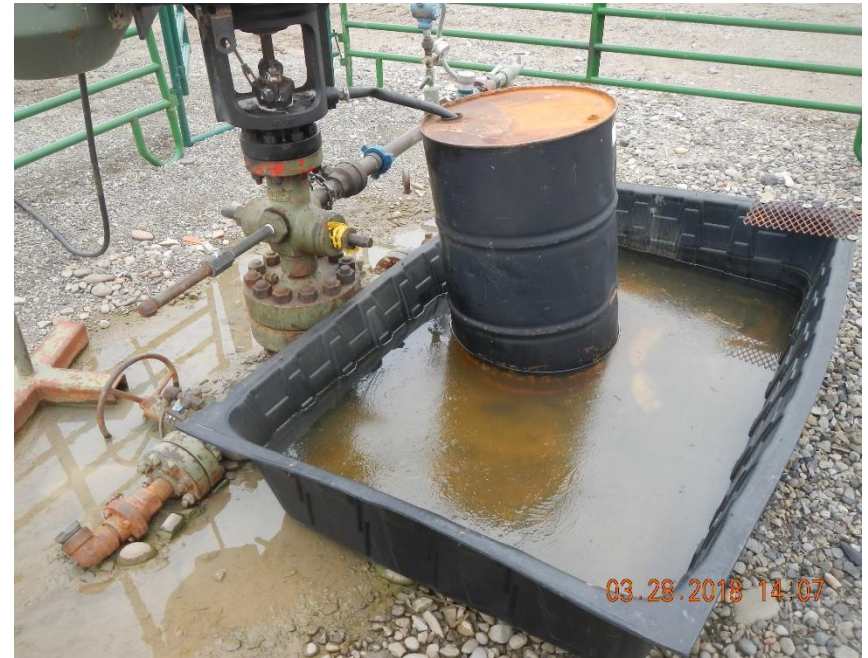
Oil drain to 55 gal. drum in secondary containment.
