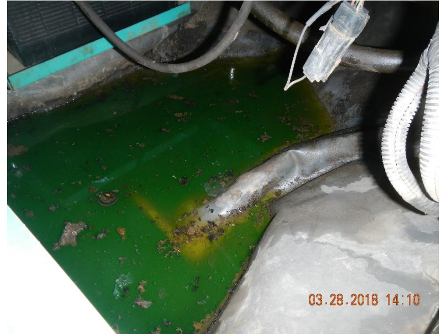
Antifreeze leak under generator engine.
