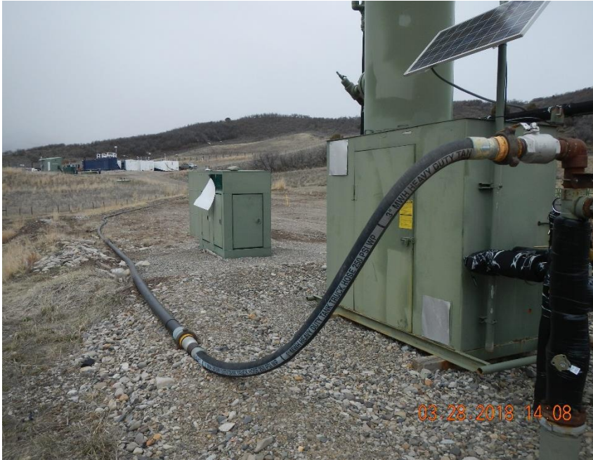
Vertical separator with produced water line.
