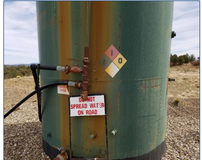
Photo 4. No tank capacity posted on tank
