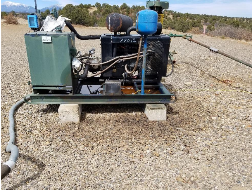
Photo 3. Stained soil around prime mover
