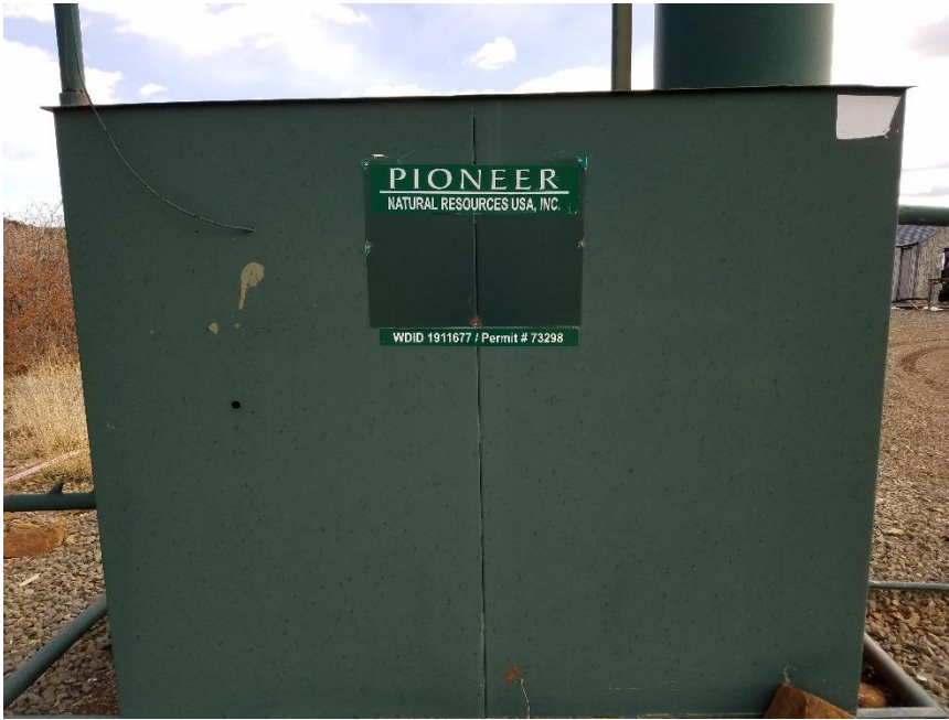
Photo 1. No location sign
