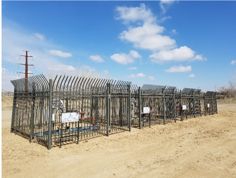
Photo 1. Wellhead looking north
