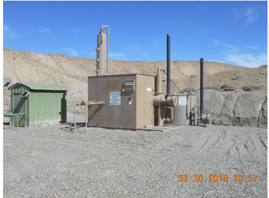
Meter housing, Separator and tank.
