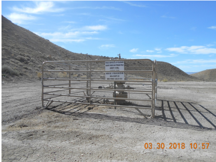
Wellhead with sign and fence
