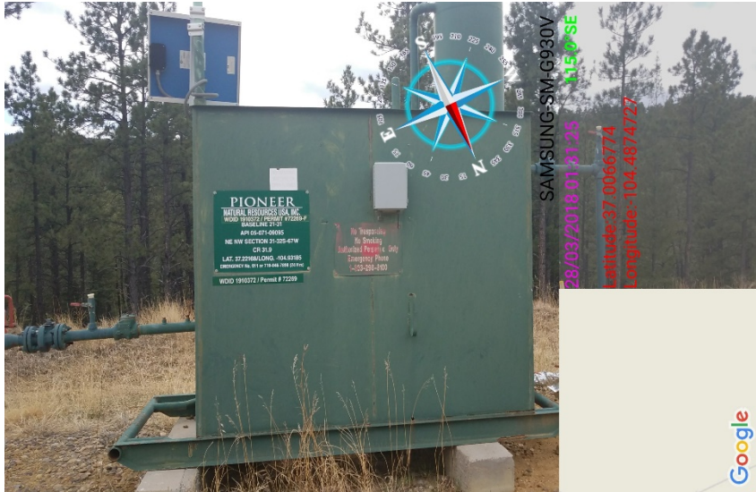
Location Sign @ Meter House
