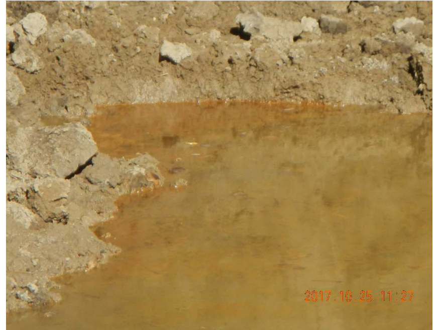
Condensate floating on water in the excavation
