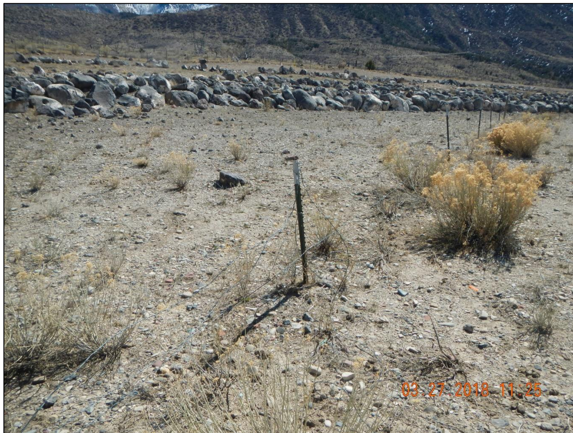
Fence is in disrepair.
