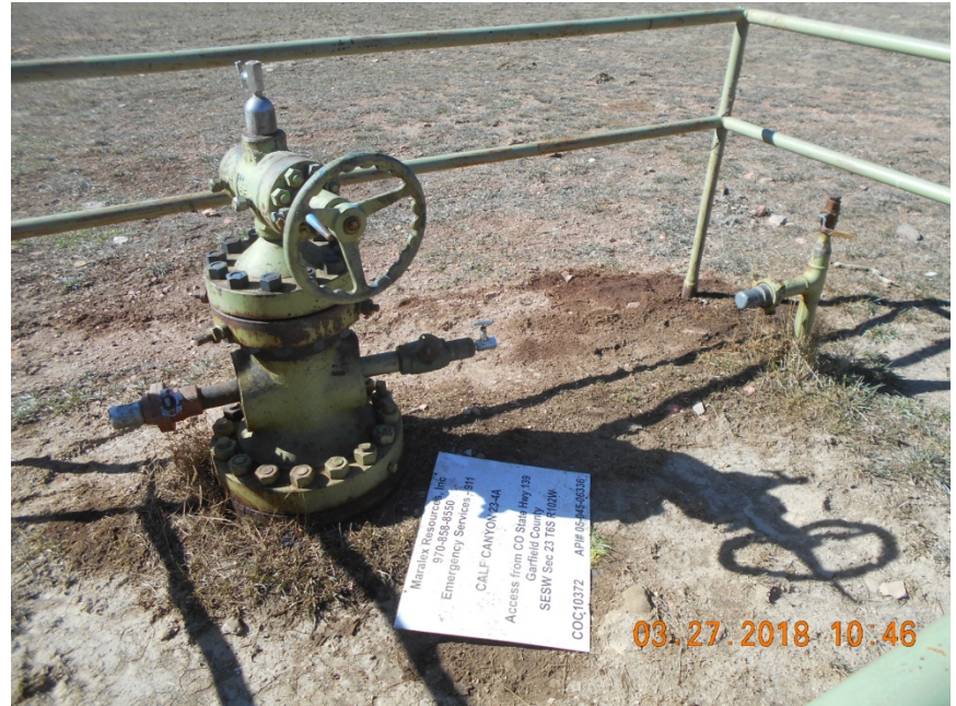
TA Wellhead with sign and unused riser.
