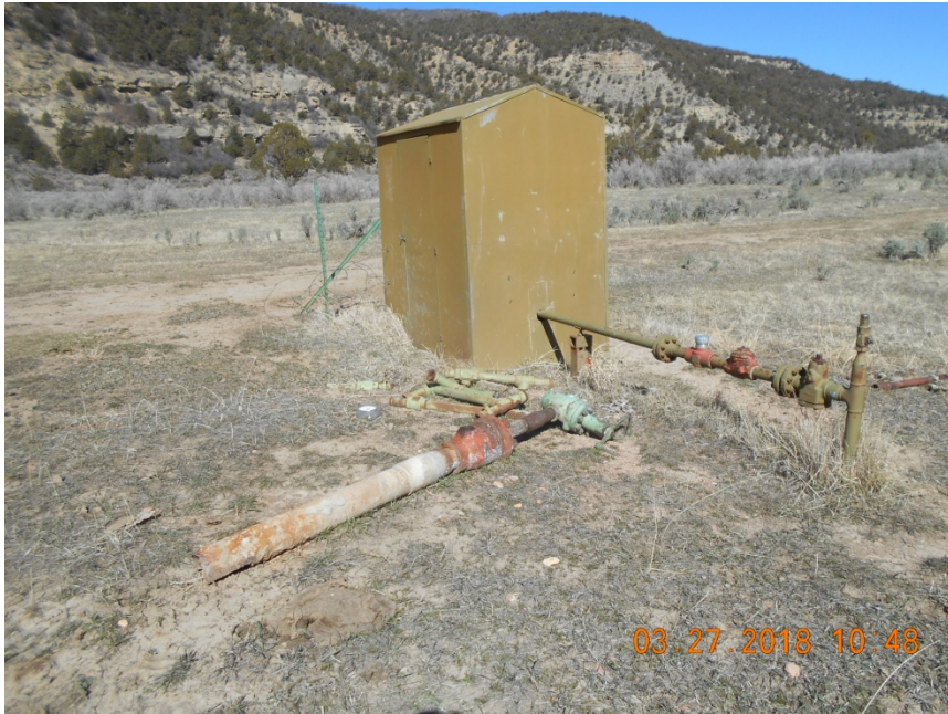
Meter housing. Cutoff wellhead from PA well (045-06134)
