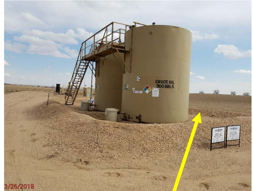
Tank Battery facing SE. Berms appear inadequate for containment.
