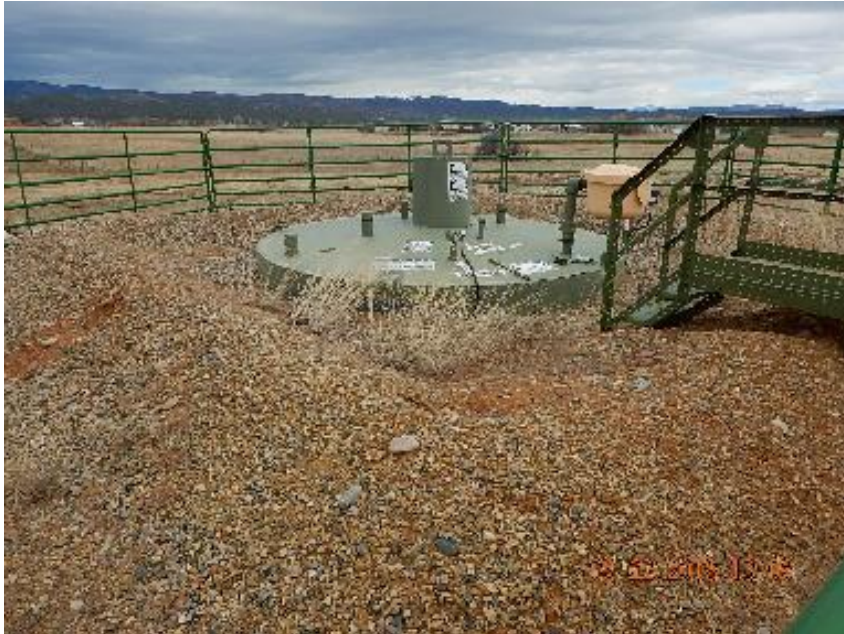
Photo 5: Dried grass noted inside containment berms.
