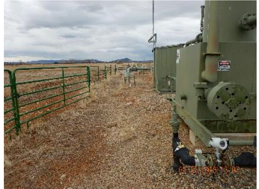
Photo 6: Dried vegetation noted inside production equipment fencing.
