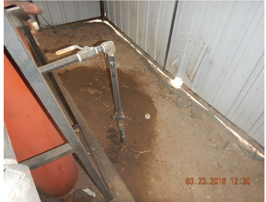
Photo 4: Stained soil in engine house
