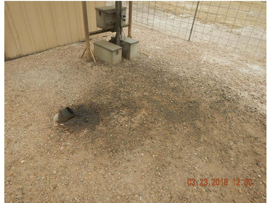
Photo 3: Stained soil at exhaust
