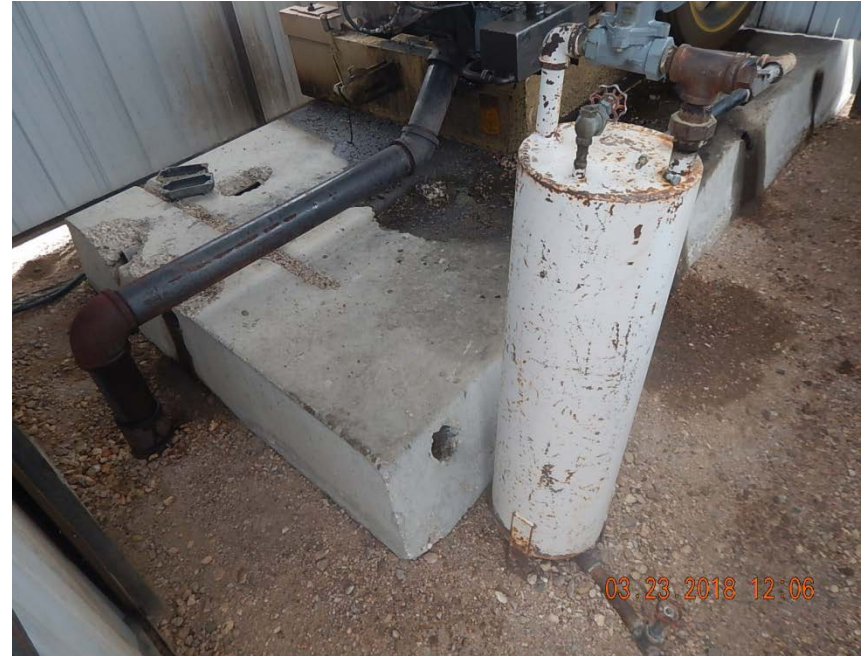
Photo 4: Stained soil at engine
