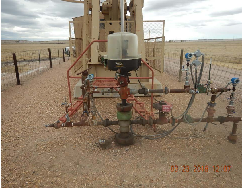
Photo 1: Wellhead, looking E
