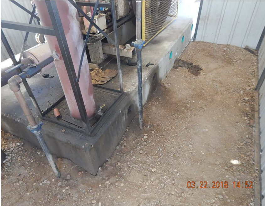
Photo 3: Stained soil at engine
