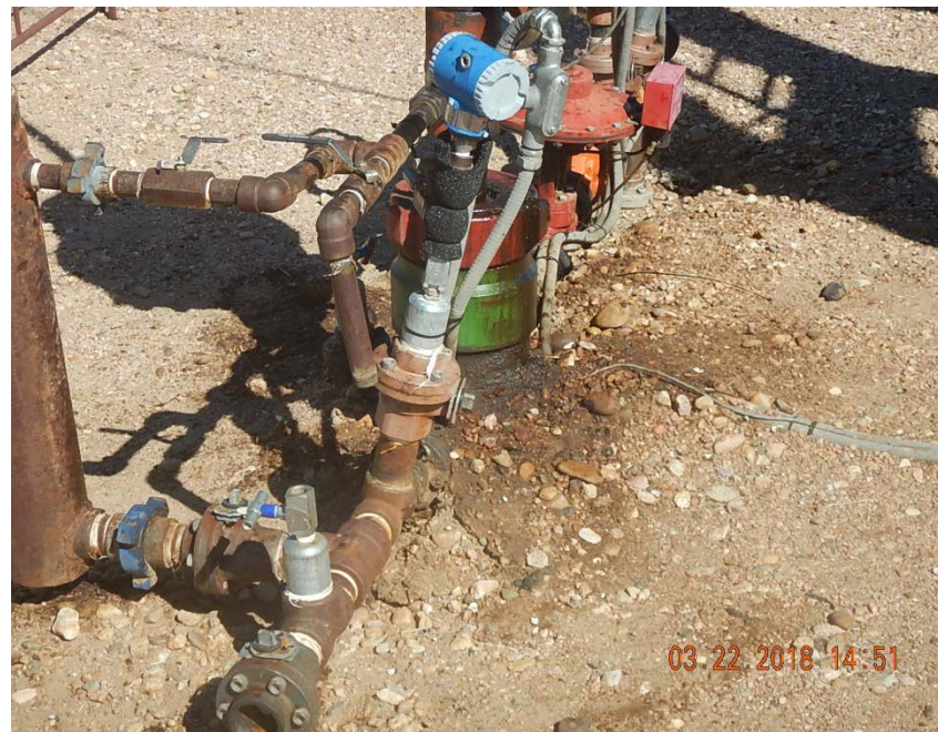
Photo 2: Stained soil at wellhead
