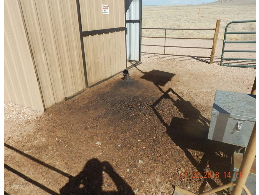
Photo 4: Stained soil at exhaust
