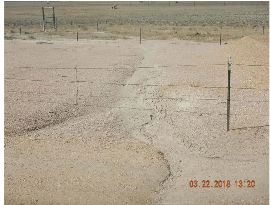
Photo 4: Stormwater erosion from center of location, looking NW
