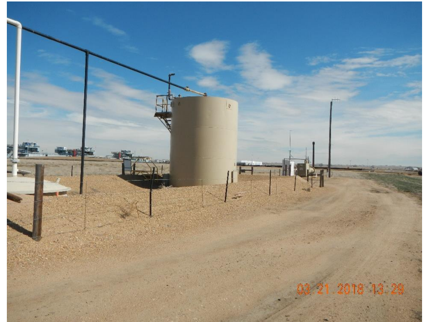
Tank battery site from SW view
