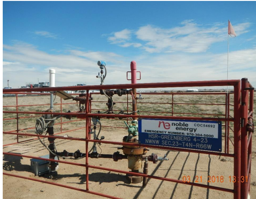
Wellhead and signage from SW view
