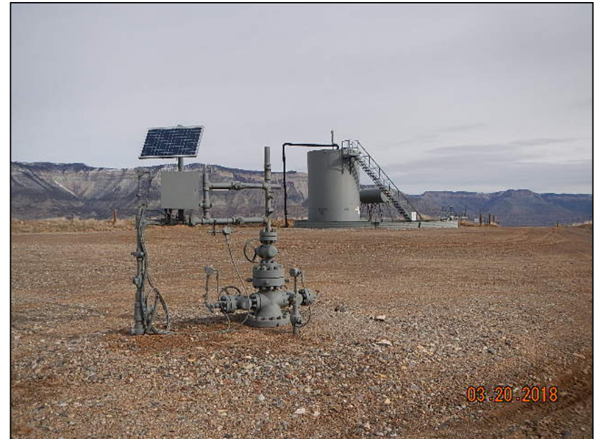
Photo 2. Wellheads and tanks.
