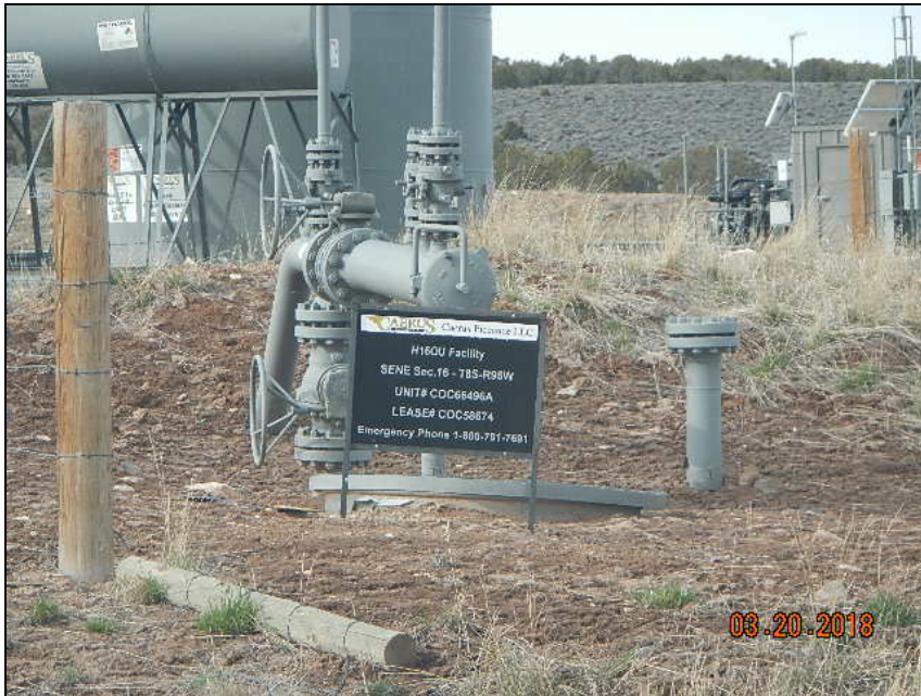
Photo 1. Sign at entrance and equipment on location.
