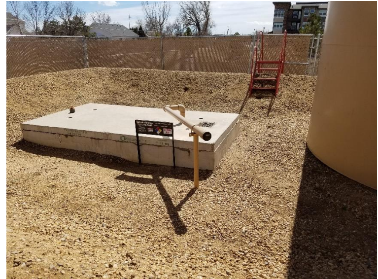
Photo 2. TANK SIGN W/ NO CONTENT LABEL
