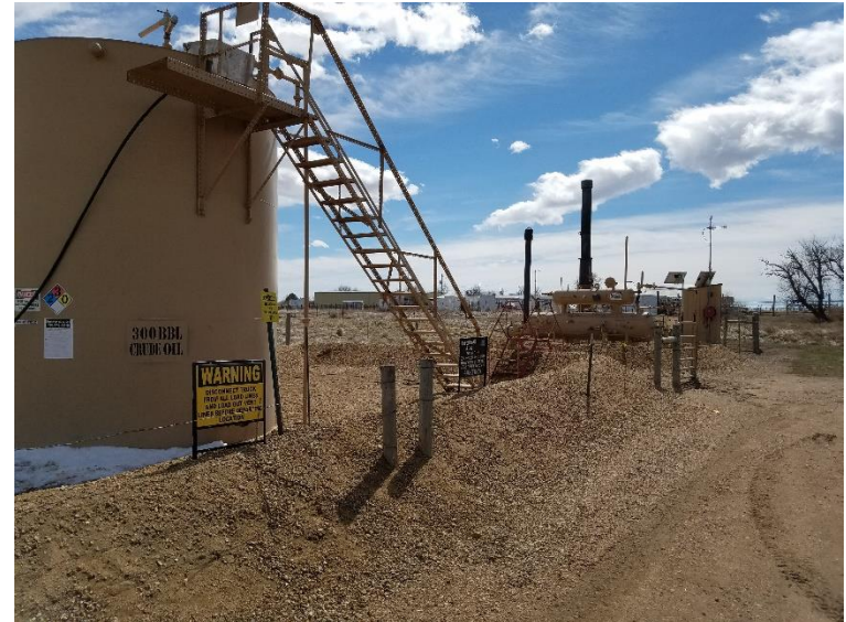
Photo 2. TANK W/ FIRED VESSEL
