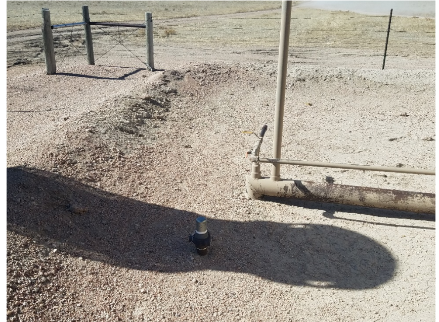
Photo 4: Unused 2" plugged riser
