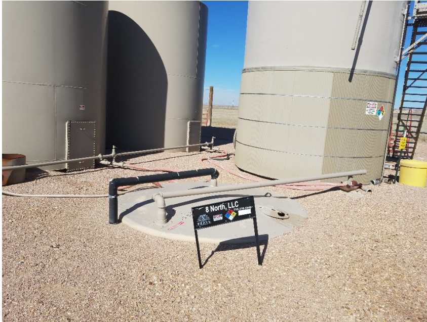
Photo 5: Water vault capacity not shown
