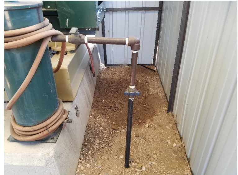
Photo 2. stained soil in engine house
