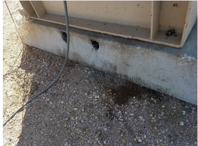
Photo 4. stained soil at base of pumpjack
