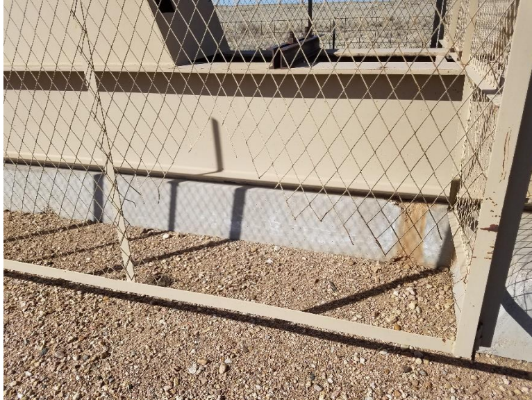
Photo 5. whole in fence around pumpjack
