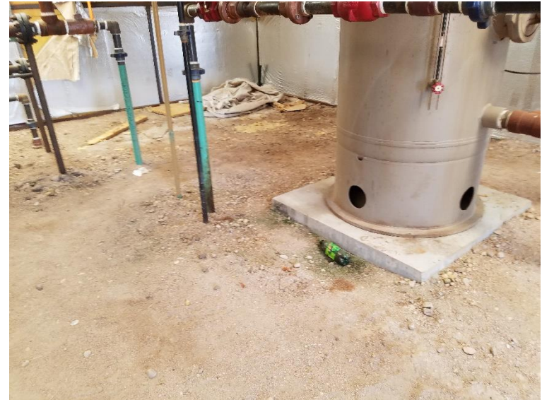
Photo 8. trash in treater house
