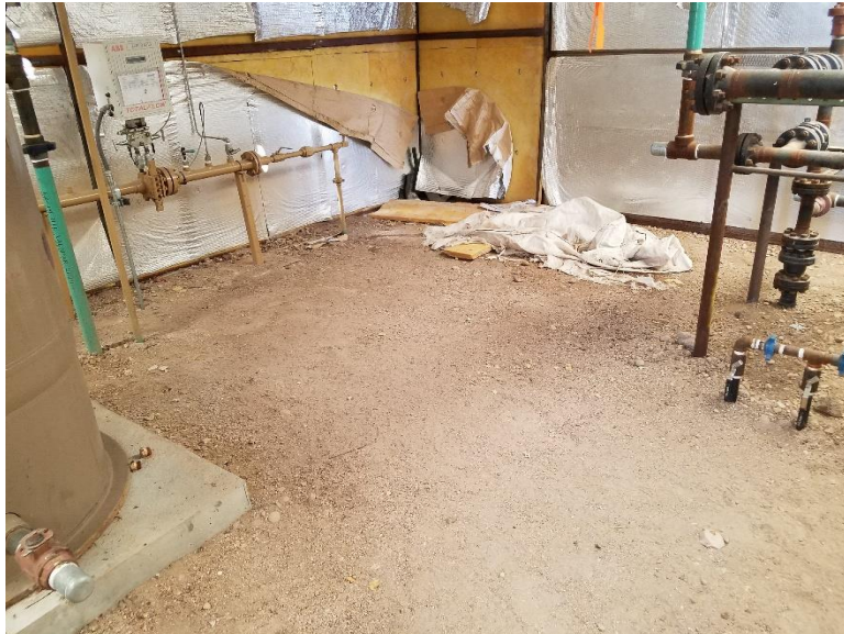
Photo 9. trash in treater house
