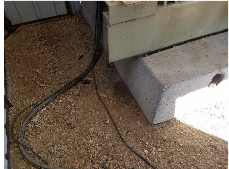
Photo 6. stained soil at base of engine
