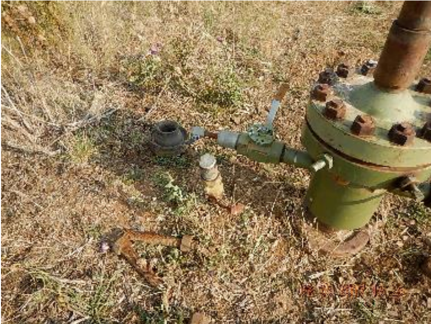
Photo 3: Debris at wellhead. Previous inspection
