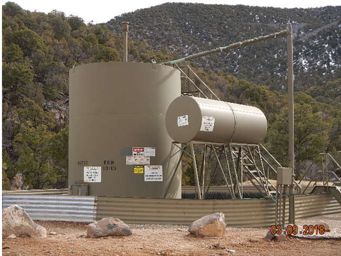
Photo 1. Methanol tank has been stood back up.
