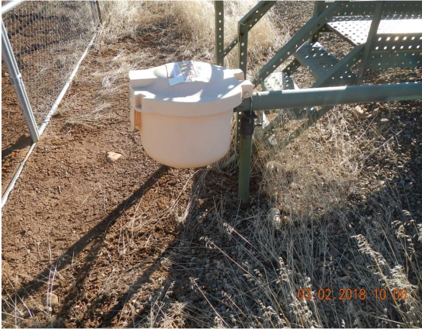
Drip pot on load out line.
