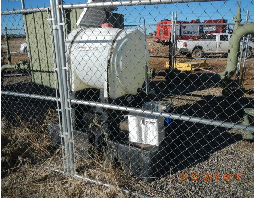
Label on container is faded and worn. No NFPA placard.
