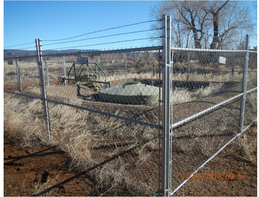
Weeds present within secondary containment berm.
