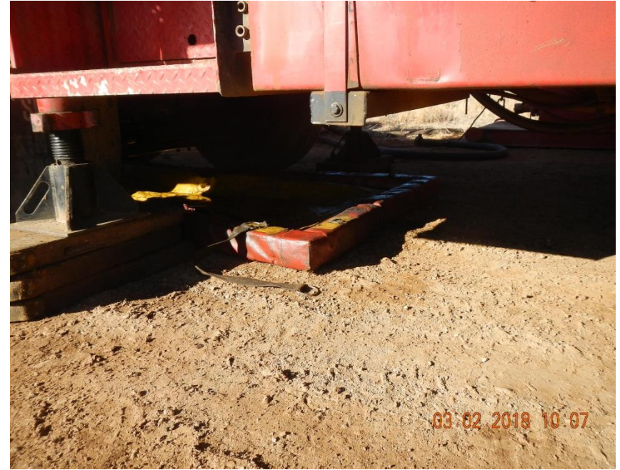
Spill prevention underneath rig engine.
