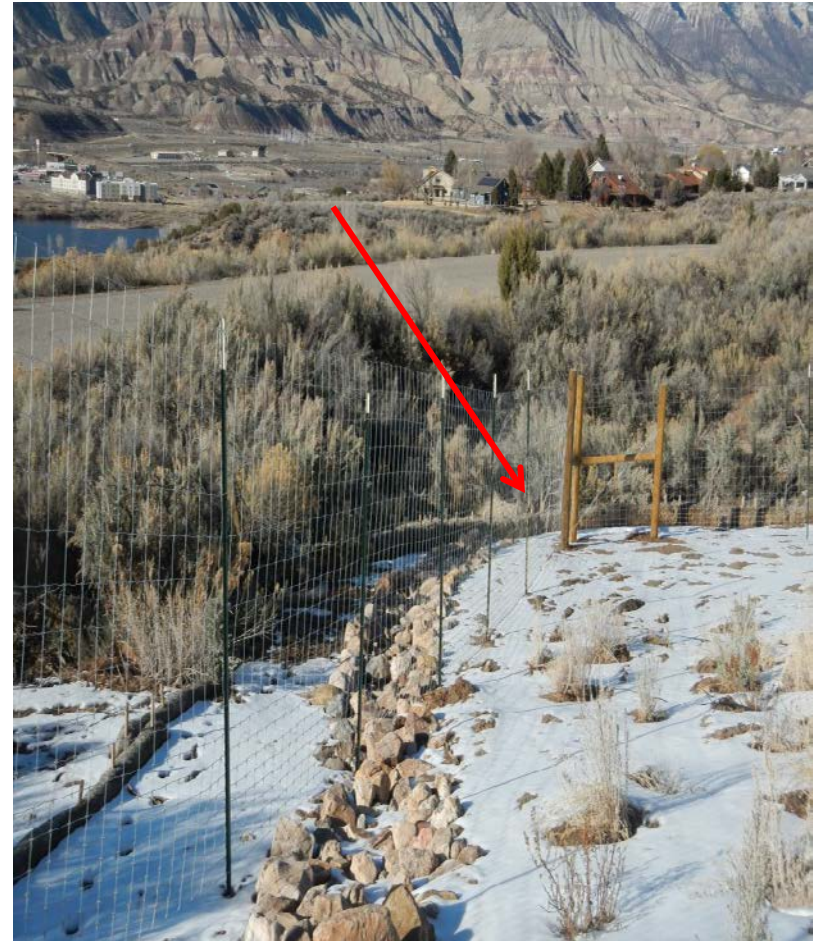
Photo#6: Arrow indicates where BMP Failure (Photo #5) is located; on outside of Fence & backside of straw bales.
