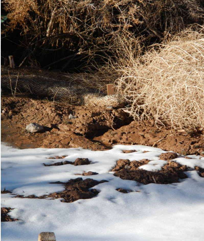
Photo#5: Area where Stormwater is starting to undercut Wattles. *
