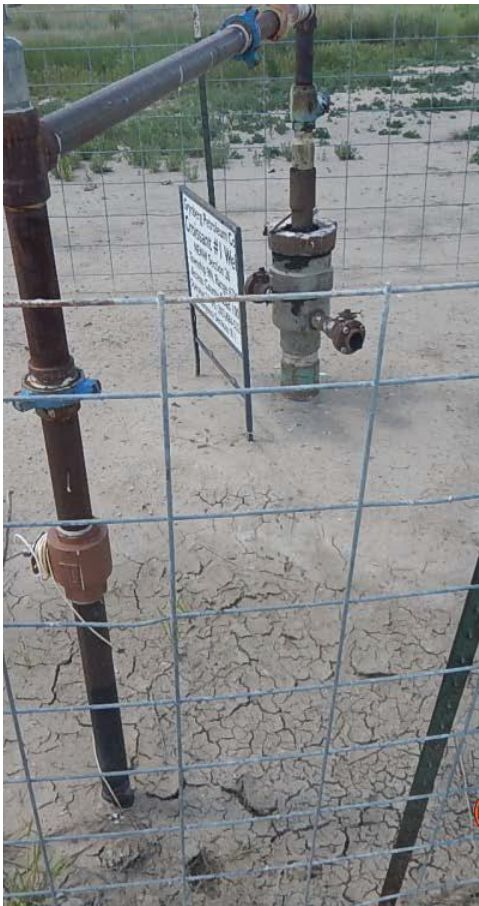
Photo 1 Photo from previous inspection, bradenhead not exposed at surface.
