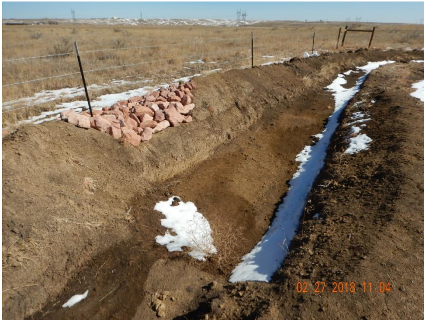
Photo 11. Photo taken from the northeast sediment trap, facing East. Sediment trap appears to be in proper functioning condition. No sediment discharge from location was observed.
