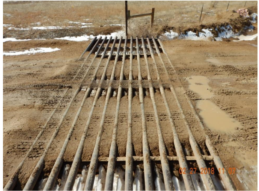
Photo 4. Photo taken from the tracking pad device at the entrance of the well pad location, facing West. Appears maintenance is required as sediment has accumulated in the tracking pad device and is no longer properly functioning.
