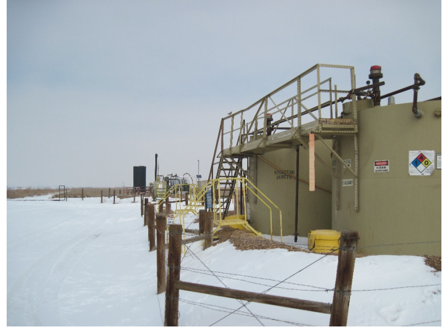
BATTERY PROD EQUIPMENT
