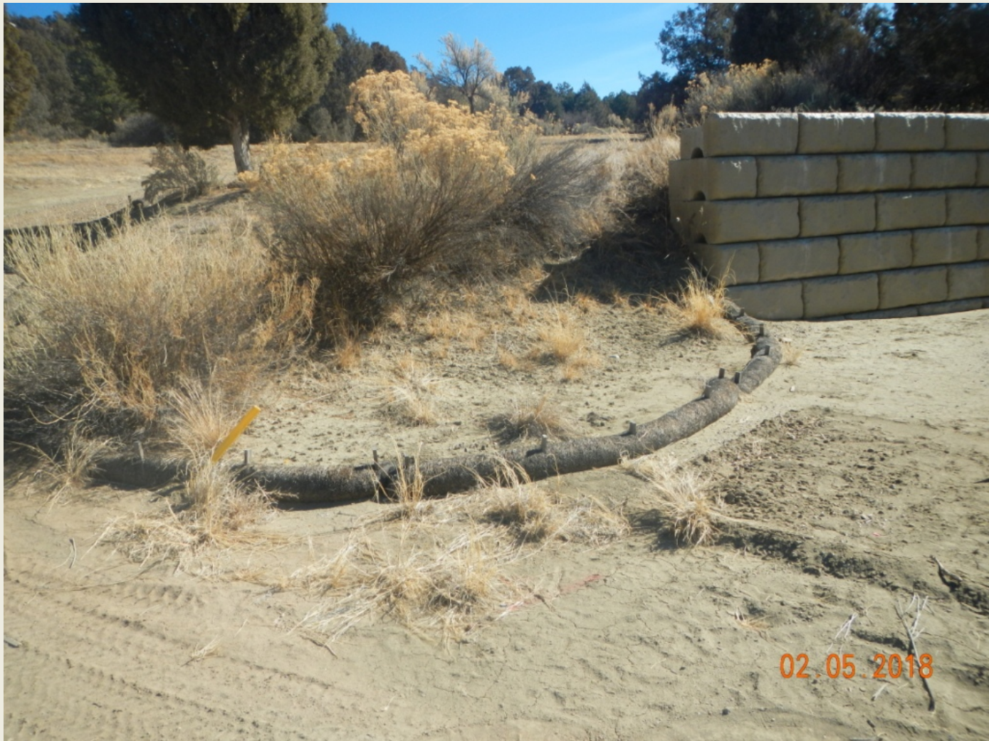
Photo 4. View of stormwater controls south of the access entrance. Appear to be functioning.
