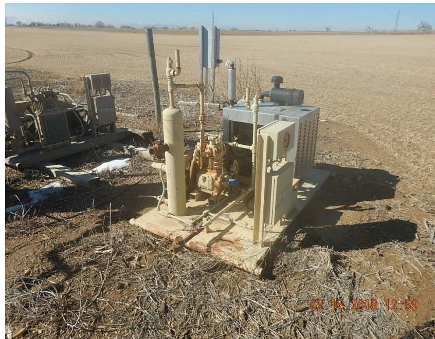
Photo 4: Unused compressor noted in prior inspection
