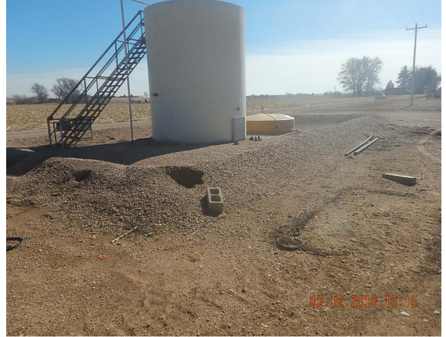
Photo 6: Unused equipment removed, some debris remains. Burrows in berms.
