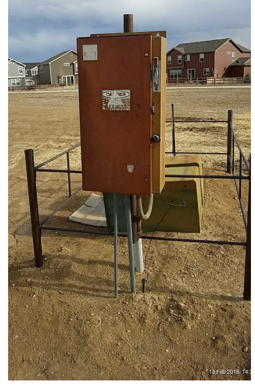
Photo 3 Pumping Unit Controller
