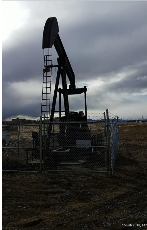
Photo 1 Wellhead API 05-123-0873 With Pumping Unit
